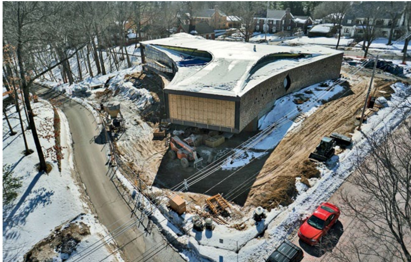
Because of the building’s boomerang shape, its cordwood walls are curved, complicating construction.
